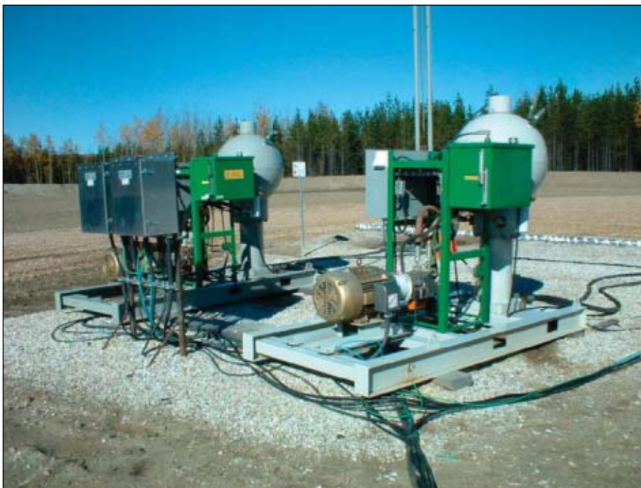
A closer view of the Trident installation shows the control-power systems for the two hydraulic rod pumps. The cylindrical vessels are the accumulators. The skids also include hydraulic pumps and control boxes (Fig. 3).
