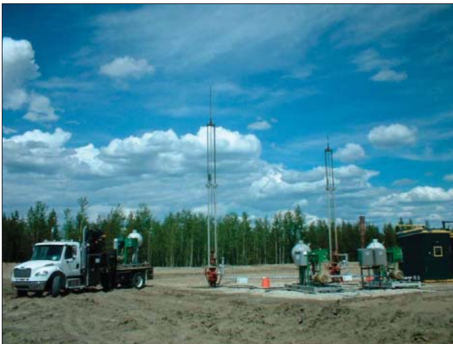
Trident Exploration Corp. installed two of the new hydraulic rod pumps on wells near Swann Hills, Alta. Two hydraulic cylinders on each pump string pull the rods up, while gravity pulls the rods under control back into the well and recharges the pressure accumulators (Fig. 2).
