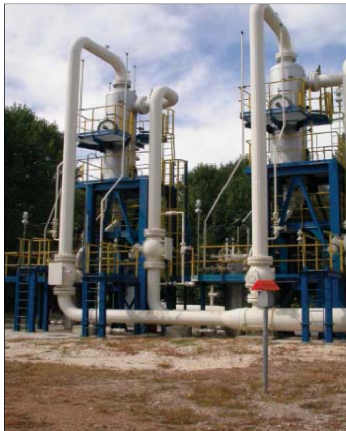
In order to protect its downstream system from black powder, DEPA installed two cyclone (centrifugal) filtration facilities at the start of its network next to the Bulgarian border. Use of these filters enhanced the effectiveness of trap filters further downstream (Fig. 6).
